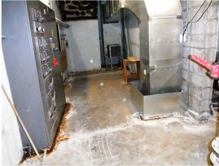
Photo 3: Crystalline salt deposits on floor slab and lower portion of walls and mechanical equipment
