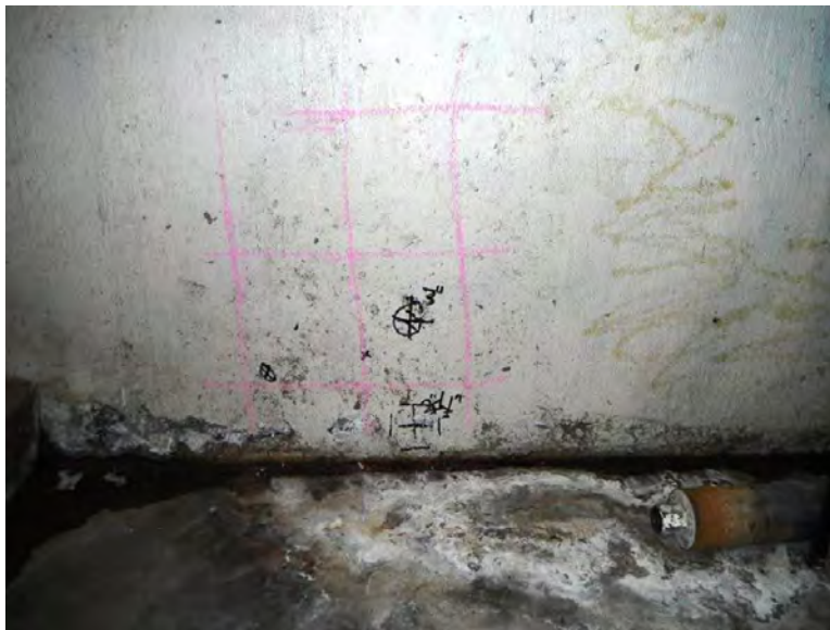
Photo 2: Crystalline salt deposits on floor slab and lower portion of walls
