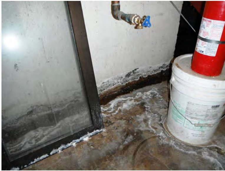
Photo 1: Crystalline salt deposits on floor slab and lower portion of walls
