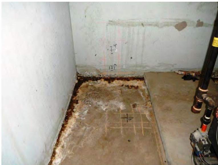
Photo 3: Crystalline salt deposits on floor slab and lower portion of walls
